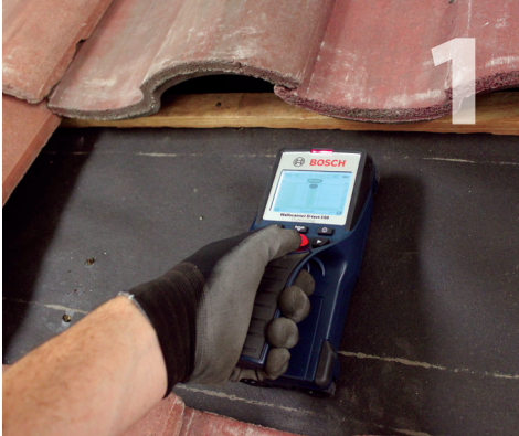
Remove the tile at selected location of the mount. Locate and mark the center of the rafter.
