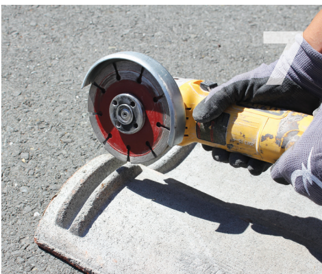
Cut a clearance notch in the weather guard lug using a grinder with a tuck point blade. Make sure the tile seats back down in its original position. Leave at least 1/4" of tile to prevent breaking through.
