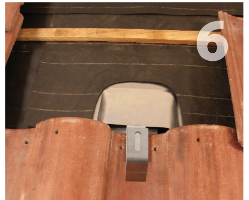
Waterproof at underlayment level according to roofing manufacturer instructions and Tile Roofing Institute Guidelines.
